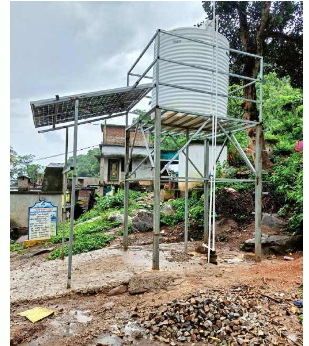
SOLAR POWERED BOREWELL WITH OVERHEAD TANK
