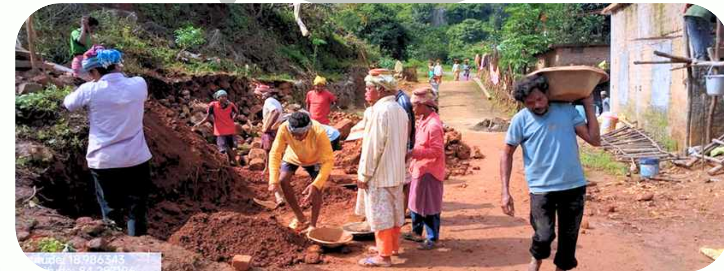
Construction of Guard Wall at South Sahi after Requesting through the VDC (10 Lakh)
