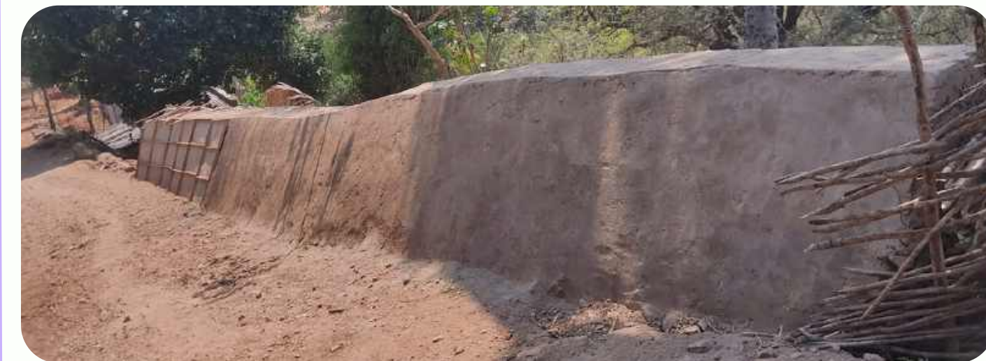
(LP 10) Construction of Guard Wall at Sana Tapanga after Requesting through the VDC (10 Lakh)
